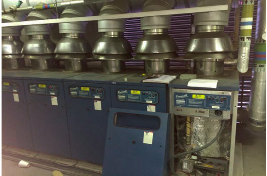
Pendle Leisure trialled RAPID BOIL™ at West Craven Sports Centre in Barnoldswick
