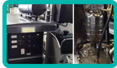
50kw Ford motor in a genset Located in Western United States
